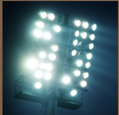
Lighting Tower Control Modules
